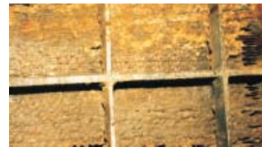
prior to cleaning
