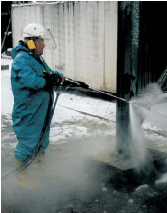
High-pressure gun with single nozzle type Form 8 for paint stripping of steel girders
